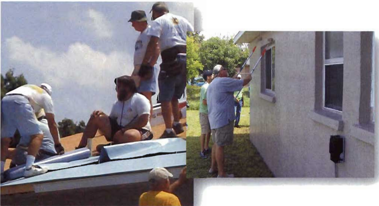
LEFT: Habitat for Humanity volunteers underlay roof in preparation for new wind resistant metal roof.
